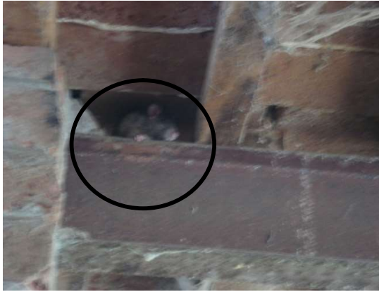
Fig. 4. Rodent found in between the girders on the roof
